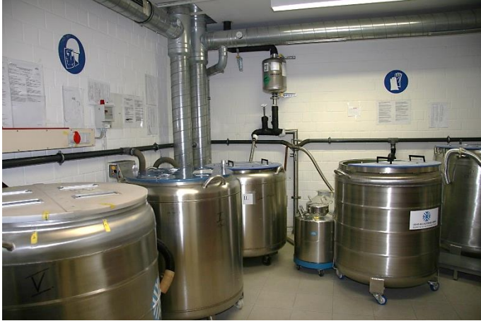
Storage in liquid nitrogen storage tanks
